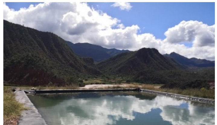
Tank for more flexible water tower management and pressurisation
